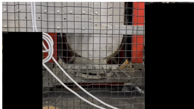
Fig. 7. Facility A lift looking from on the floor
